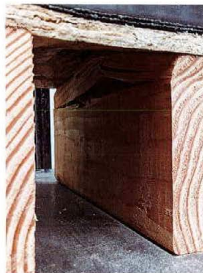
Figure 3c. Rafter view of typical failure
